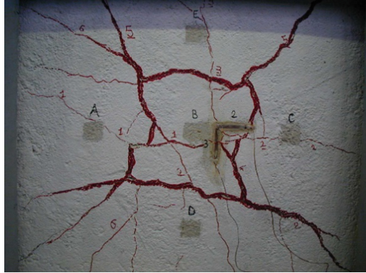
Fig. 6. Cracking at failure of plate with carbon fibres.
