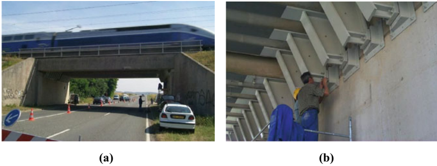
Fig. 12.5 a Overview of the viaduct during a TGV crossing; b Detail of the strengthening procedure taking place
