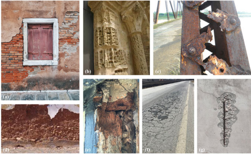
Fig. 2.1 Degradation forms observed in different materials: a render, masonry bedding mortar and brick deterioration; b sandstone alveolization; c steel corrosion; d rammed earth lack of cohesion; e timber deterioration; f bituminous mixtures cracking; g concrete spalling
