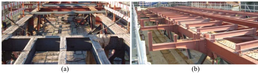
Fig. 10.11 Luiz I Bridge. Replacement of the upper-deck floor system a removal of the lightweight concrete pavement; and b installation of the new floor system
