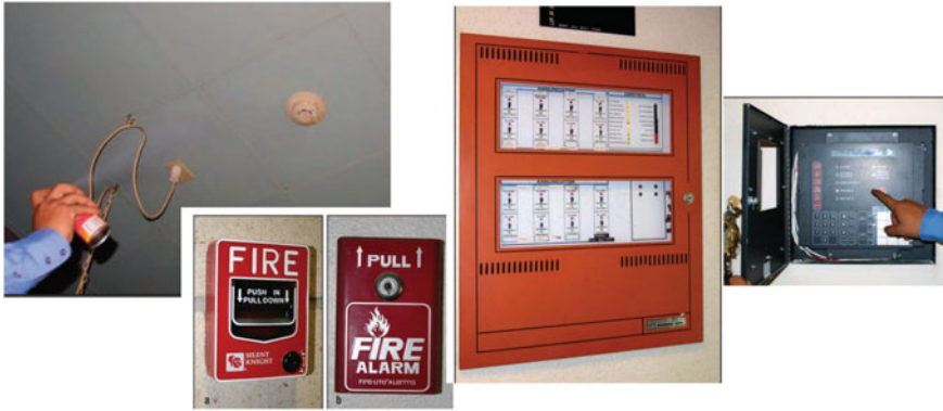
Fig. 16.5 Automatic detection and alarm systems test
