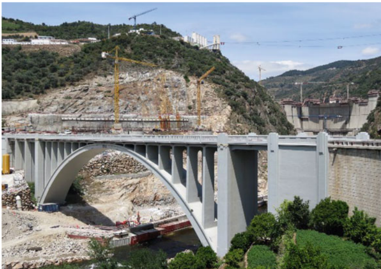
Fig. 10.16 Foz Tua Bridge and the construction site of the Foz Tua Hydroelectric Plant (2012/16)
