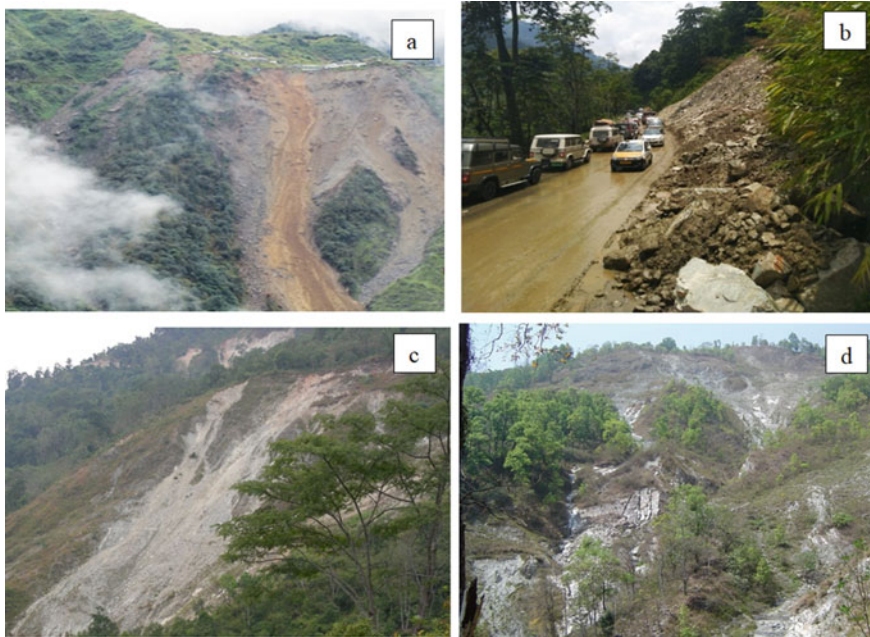
Fig. 14.3 Field photographs of landslides in the study area a Landslide near the settlement b Active landslide on the Rangpo—Namchi link road c Step slide area d Exposed old slide-vulnerable to failure
