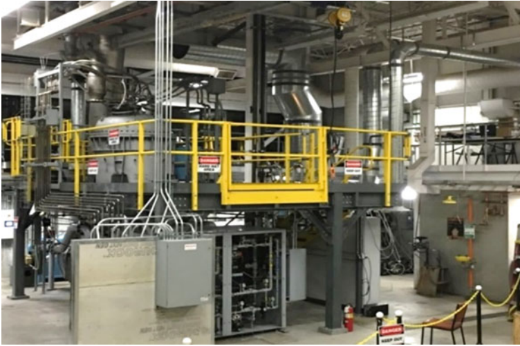
Fig. 3 The pilot plant with a flash reactor installed at the University of Utah (Adapted from Elzohiery [20])
