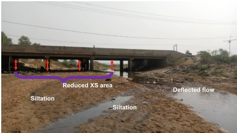
Fig. 4. Showing flow deflection, siltation and undermining of bridge abutment
