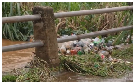
Fig. 7. Blockage of water channel with refuse. Source: Field Survey (2019)
