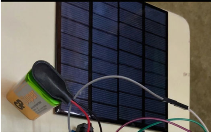
Fig. 14.4 Solar panel with battery
