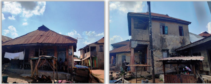
Fig. 5 Dilapidated buildings in informal settlements in Nigeria during the COVID-19 lockdown measures: ( left ) Beere area in Ibadan—5 April 2020 and ( right ) core area of Osogbo—26 March 2020. Source: Photographs by Adewale O. Yoade
