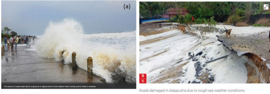
Fig. 2.2 (a) Cyclone Hudhud at Uppada beach, Andhra Pradesh. (b) Cyclone Tauktae damages the beach roads in Alappuzha, Kerala
