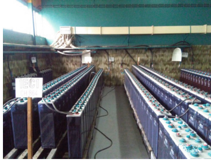
Fig. 2. Battery plant. Source TE-TO Zr, personal archive
