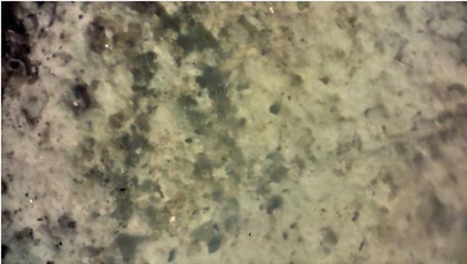
Fig. 2. The salt on the surface of the selected sample from basement under a microscope.
