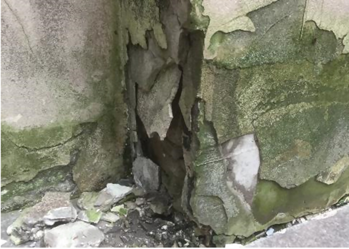
Fig. 5. Place of sampling on the surface of the facade at the level of the 1st floor.
