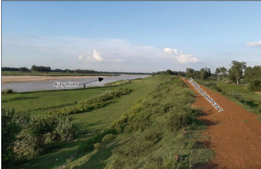
Fig. 11.1 A typical view of artificial embankment along the Ajay River near Bhedia
