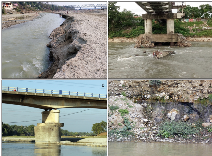
Fig. 6.10 Problems associated with channel adjustments: (a) recent incision noticed on B in December 2017, (b) signs of bed lowering on B at Matigara Railway bridge, (c) destabilized bridge pillar on M at Champasari, and (d) discharge of vadose water noticed from the black clay layer along the banks of B. Pictures were taken in December 2017 by the author. (Figure prepared by the author)
