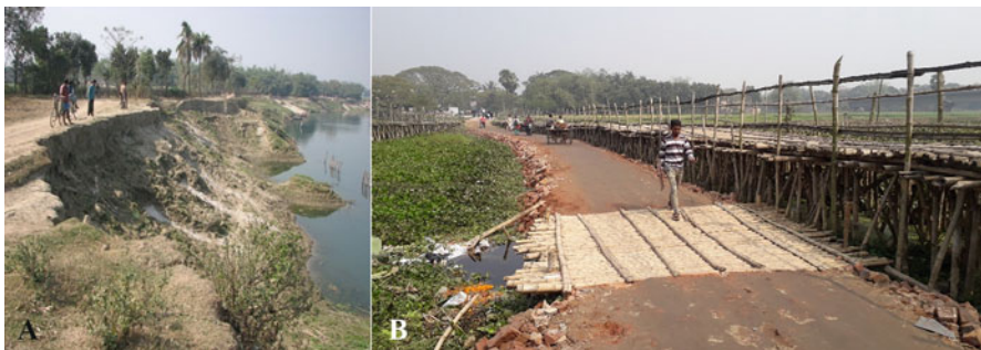
Fig. 20.10 (a) Bank erosion in middle reach and, (b) hyacinth-covered channel and cross-bandh at Karimpur-Bakshipur Ghat on the upper reach of Jalangi River
