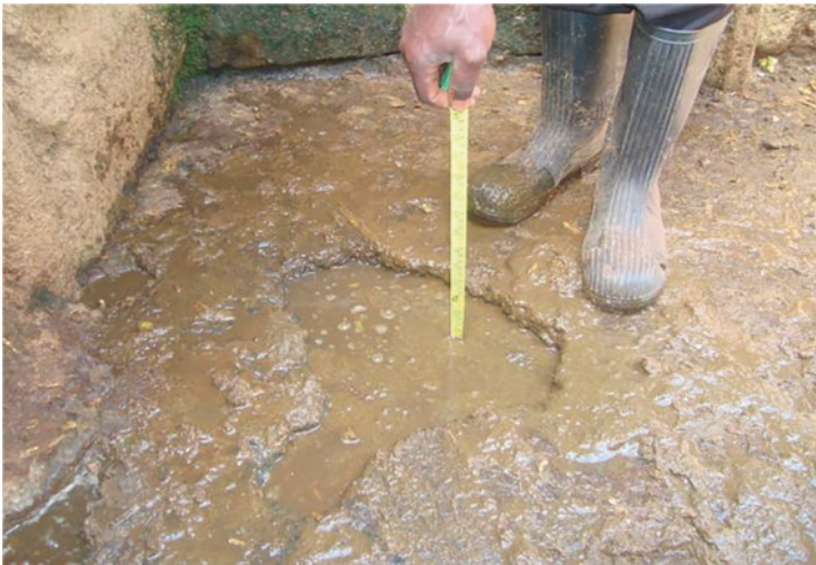
Fig. 15.6 Old and worn out concrete with an example of an excavation defect (shown by metallic tape measure dipping) in a dairy cow zero-grazing unit. The concrete edges of the defect are sharp enough to cause claw disorders. (Photograph courtesy of JW Aleri)
