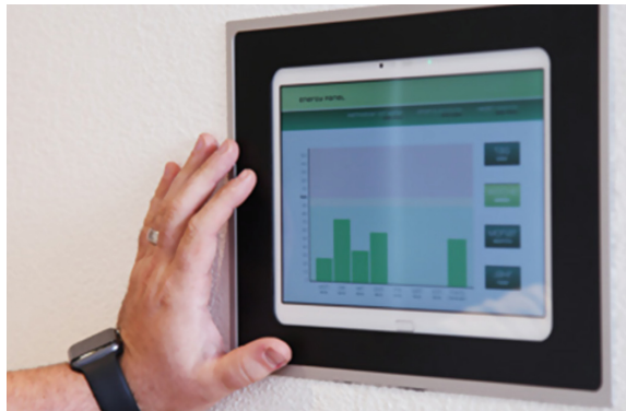
Fig. 9. Tablet with control of energy consumption ( https://www.umweltarena.ch/ ).
