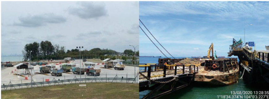
Fig. 1 (left) Excavated soil transported by dump trucks to the Staging Grounds, (right) Excavated soil loaded onto barges for transportation offshore
