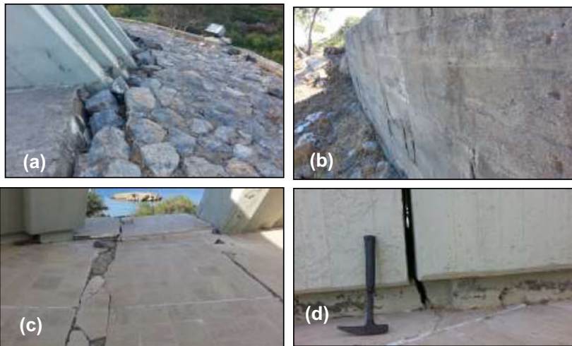
Fig. 5 Some damages observed: a. The stone pavement adjacent to the monument is separated from the monument towards the north; b. Buckling of the retaining wall by the load forcing from north to south; c. Partial subsidence formed in the Ceremony Square especially extends along the drainage channels; d. The fracture in the foundation under the two concrete joints
