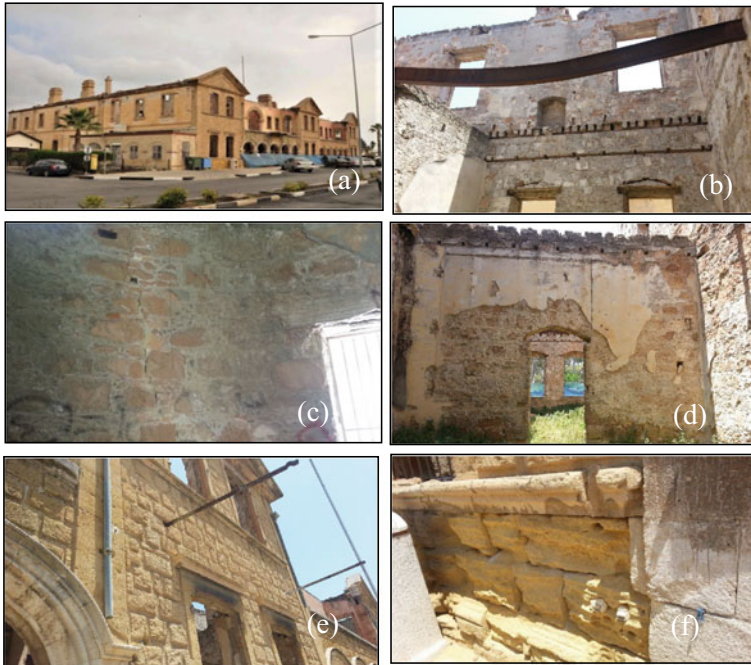
Fig. 1 Various views of the British Government building: a Present view; b Bended steel beams due to heat expansion; c Oblique cracks in the Northeastern corner extending along joints without cross-cutting the blocks; d All wooden beams, ceilings and flammable materials were burned, interior gypsum plasters were unwrapped; e Rectangular building blocks used for exteriors are in good conditions; f On the southern front of the building 5–10 cm deep carvings formed by alteration in the 75–80 cm interval above the ground
