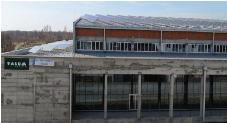
Fig. 7 Current position of the PV modules
