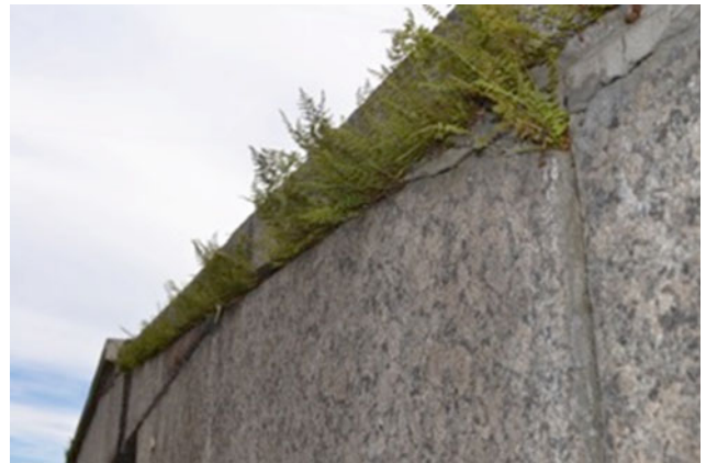
Fig. 26 Growth of ferns on a deteriorated granite facade. Exchange building. St. Petersburg
