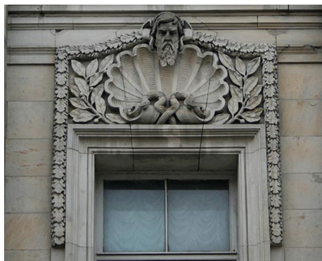
Fig. 5 Fragments of the carved decoration of the facade of the building of the former Naval Academy (11th line V.O., D. 8)
