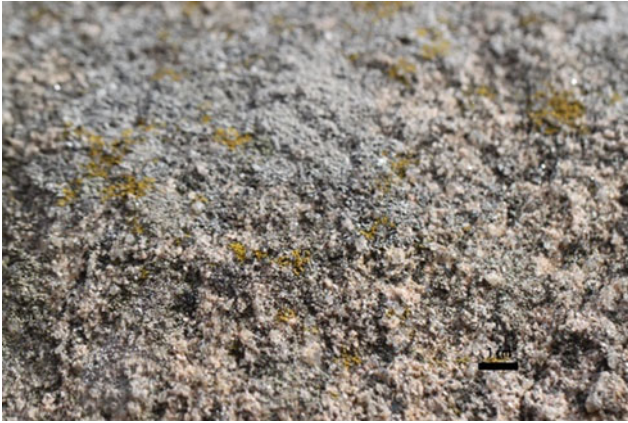
Fig. 22 Crustose lichens on the surface of granite. Granite embankment. St. Petersburg
