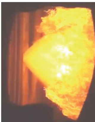
Fig. 5. Fuel oil combustion in the furnace of a power-plant boiler using a pneumo-hydrovortex nozzle
