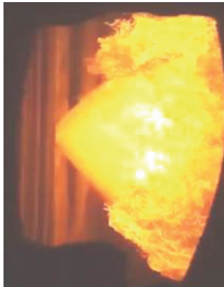
Fig. 5. Fuel oil combustion in the furnace of a power-plant boiler using a pneumo-hydrovortex nozzle
