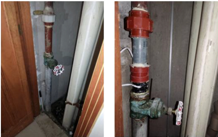
Fig. 2. Flowmeter IoT installed in the administrative building of the university
