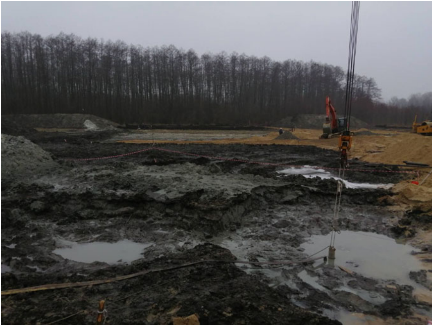
Fig. 5 A photo of a typical wetland site in the process of work before the installation of a drilling rig for the construction of an operational inclined-directed well with a depth of more than 5000 m
