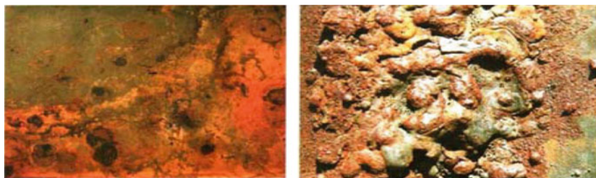
Fig. 2 Oxygen corrosion of metal
