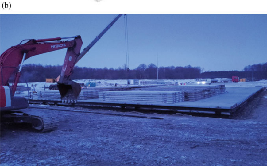
Fig. 13 Scheme of loading the foundation slab (a) and photo of the loaded slab (b)
