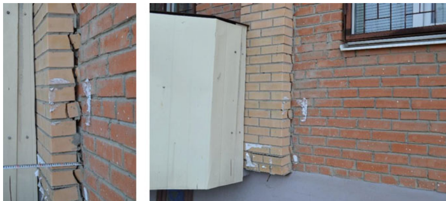
Fig. 1 Exfoliation of brick pilasters from the walls
