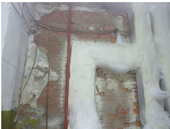
Fig. 2 Local destruction of the internal walls and plaster within the technical areas
