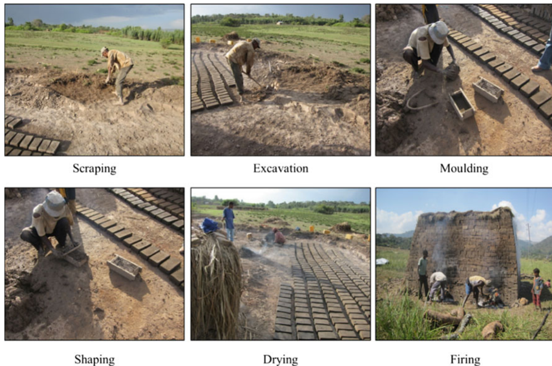
Fig. 12.3 The local brick making process in the Gilgel Gibe catchment, Southwestern Ethiopia (Source Photo by Alemayehu Regassa)
