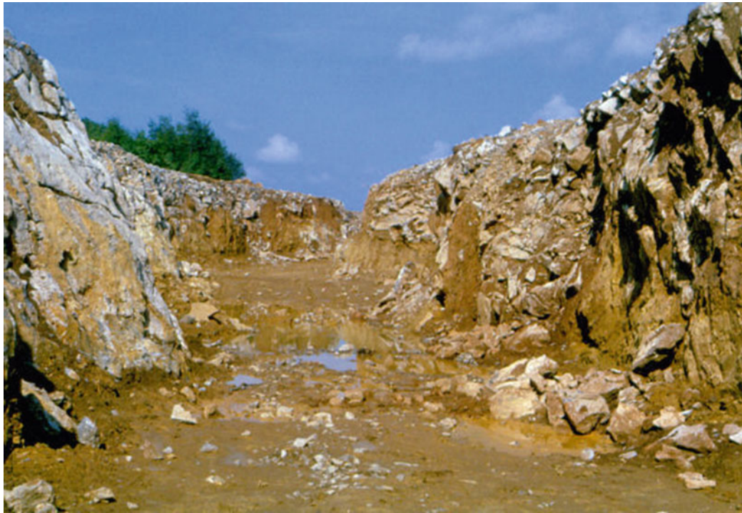
Fig. 1 During the motorway construction, a softer sediment was discovered among limestones at the level of the future roadway. To preserve static stability, the sediment was removed, which revealed the bottom part of a cave passage—an unroofed cave
