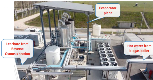
Fig. 2. Evaporation plant: top view [credits: NBT Bulgaria EOOD]
