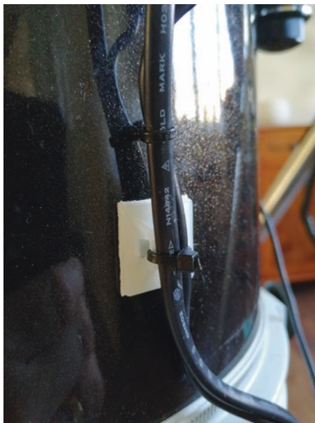
Fig. 8.54 Self-adhesive pads and Tie wraps
