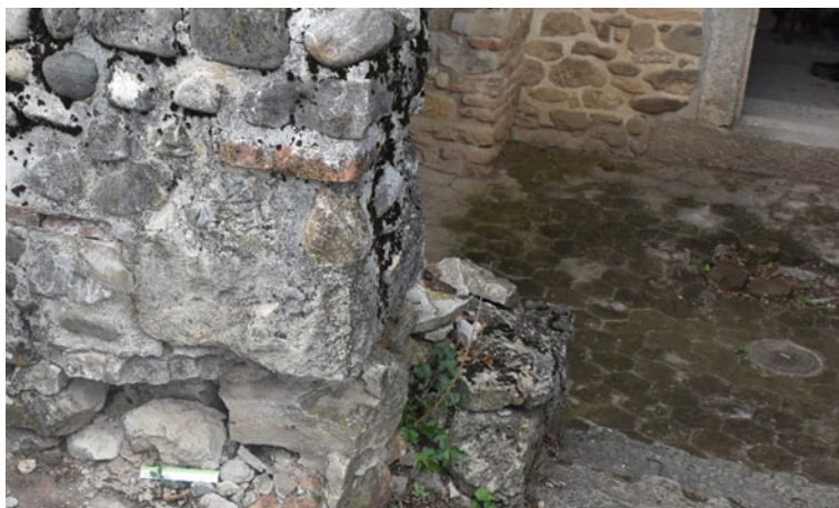
Fig. 18.3 Sampling position, masonry mortar sample Br1, late Roman tomb in Brestovik (Photodocumentation of the MoDeCo2000 project)
