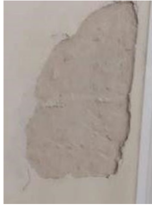
Fig. 14.8 Detailed view of one of the pathologies on the ceiling
