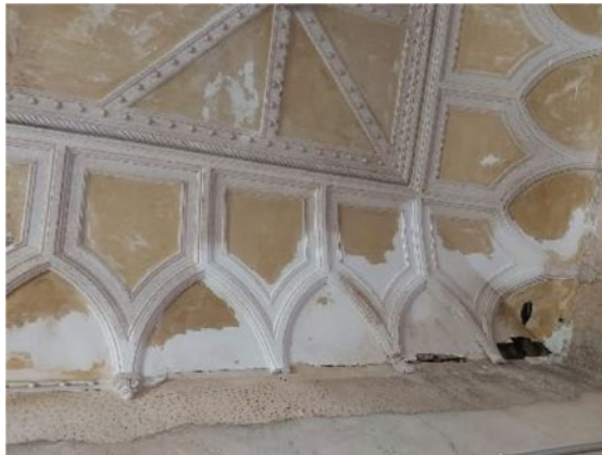
Fig. 14.7 Detailed view of some of the pathologies identified on the ceiling of the noble staircase and in other adjoining rooms
