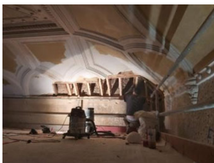
Fig. 14.10 Detailed view of the structure of the intervention roof, in noble staircase
