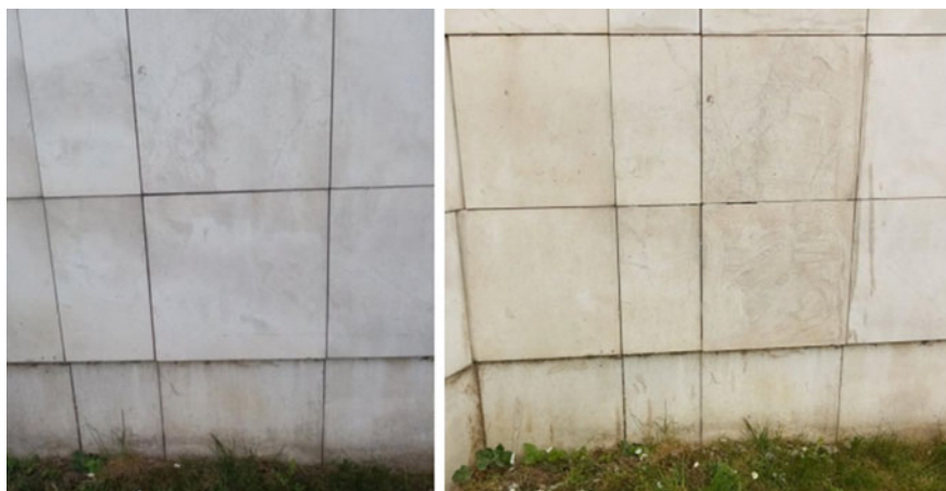
Fig. 17.6 Trial surface before treatment (left) and after treatment with the soaps (right photo, 2.5% Schmutzlöser—left slab, 10% Schmutzlöser—middle slab, 33% Kiehl Li-Ex—right slab)
