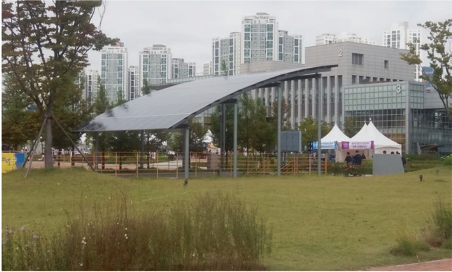
(a) Another Solar PV plant with 90 panels capacity installed at Incheon National University
