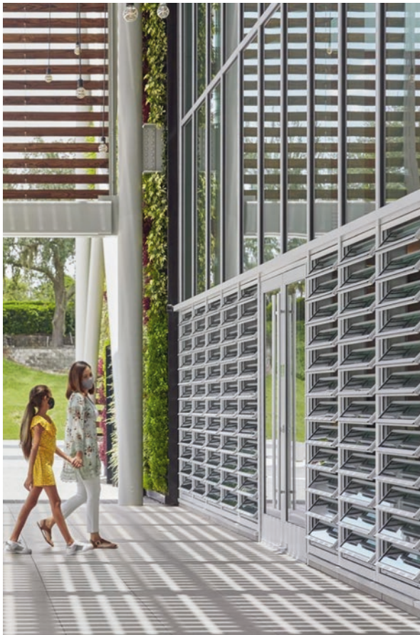
Fig. 37 Operational “jalousie windows” and wood louvers are combined to provide shade and allow for natural ventilation when desired. (Credit: Kate Joyce Studios, McDonald’s Flagship—Orlando, Ross Barney Architects, 2020)
