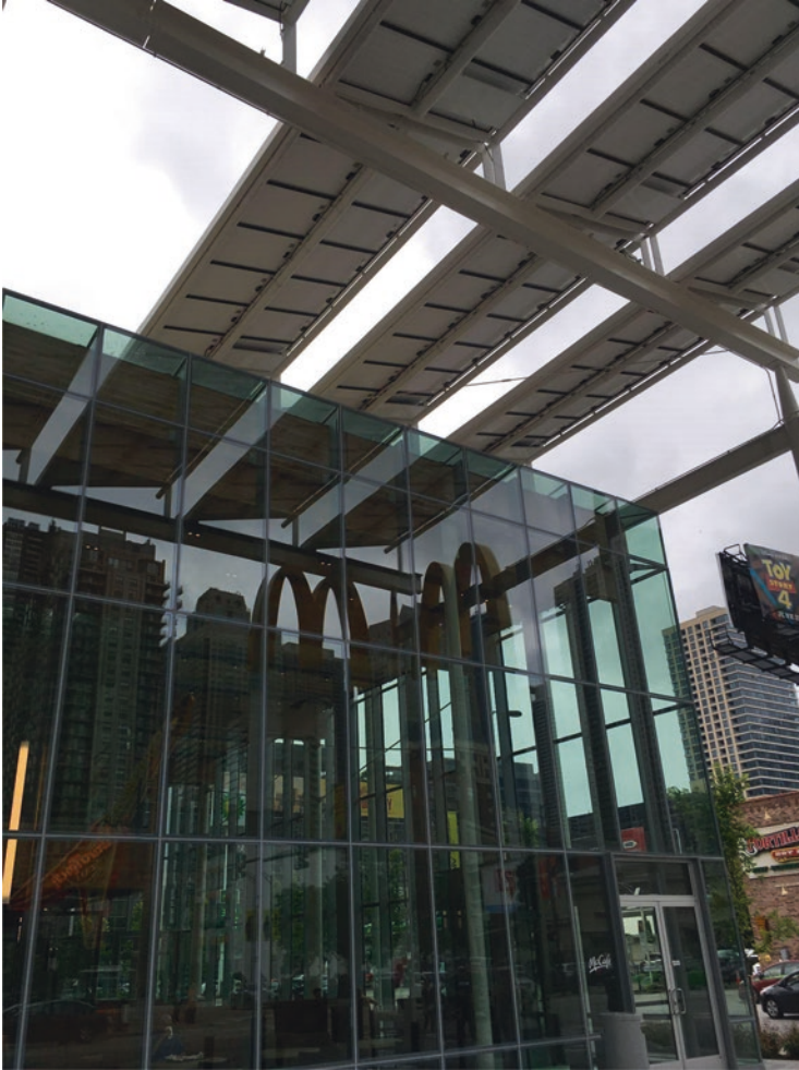
Fig. 49 A VS-1 vertical facade system curtain wall allows for natural light to enter interior spaces and views of the outdoors from the inside. (Credit: David Thaddeus)
