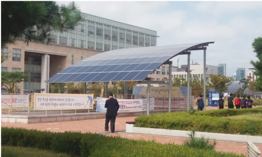
(b) A close up view of two arrays of 180-solar panels, each 90 PV panels installed at INU
