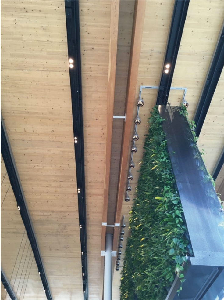
Fig. 51 Exposed timber roof deck elements can be seen from the interior dining area. (Credit: David Thaddeus)
