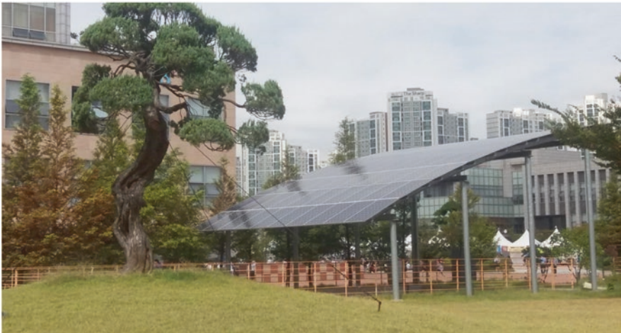
(b) View of a 180-solar PV plant installed at Incheon National University (INU) campus
