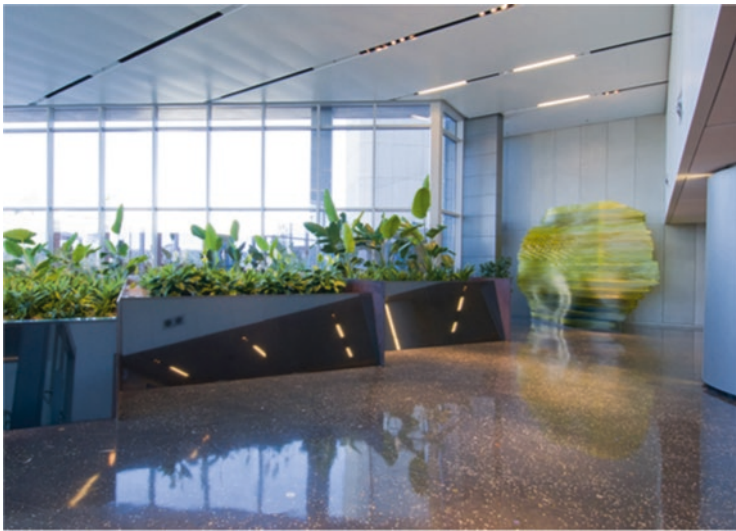
Fig. 65 The “Living Machine” mimics an interior garden while working to cycle wastewater. ( https://www.mayerreed.com/portfolio/port-of-portland-headquarters-parking-garage/ )
