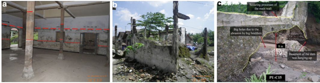
Fig. 17.14 Lahar impacts in the Kali Putih river valley. a Interior of a large building in Sirahan showing the inundation lines from the flow and deposit (red dashed lines); some damage was caused to the building exterior, and the building has since been emptied (Photo credit: S. Jenkins). b A destroyed building showing failure of the masonry infill walls within a reinforced concrete frame and some remaining deposit inside; flow direction was
