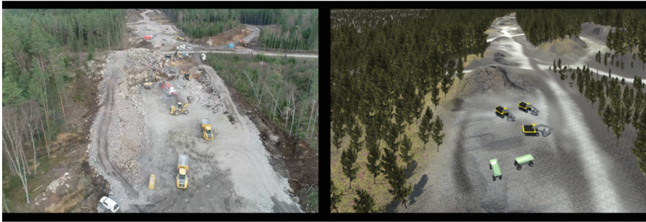
Fig. 3. Screenshot from the camera drone video used to generate the virtual scene and the corresponding 3D virtual environment.
