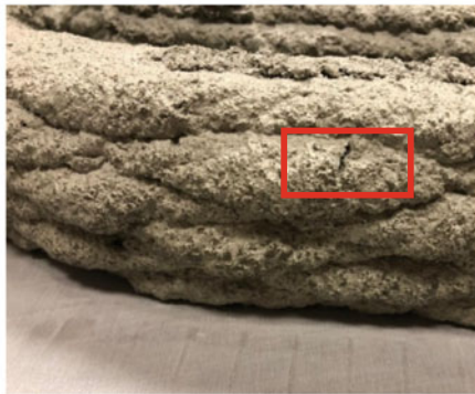
f) shrinkage cracks at local areas
