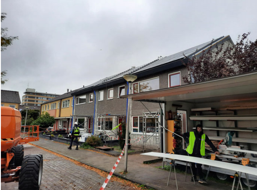
Fig. 1 Testcase houses of the INDU-ZERO project in Enschede, The Netherlands under redevelopment. Photo: Jacob Cornelis Bazen
