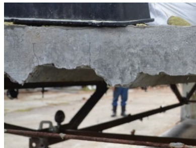
Fig. 9. Cracks in a slab (KSB-3)
