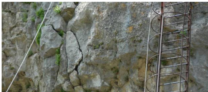
Fig. 8 Small size rockfall in the lower portion of the pillar
