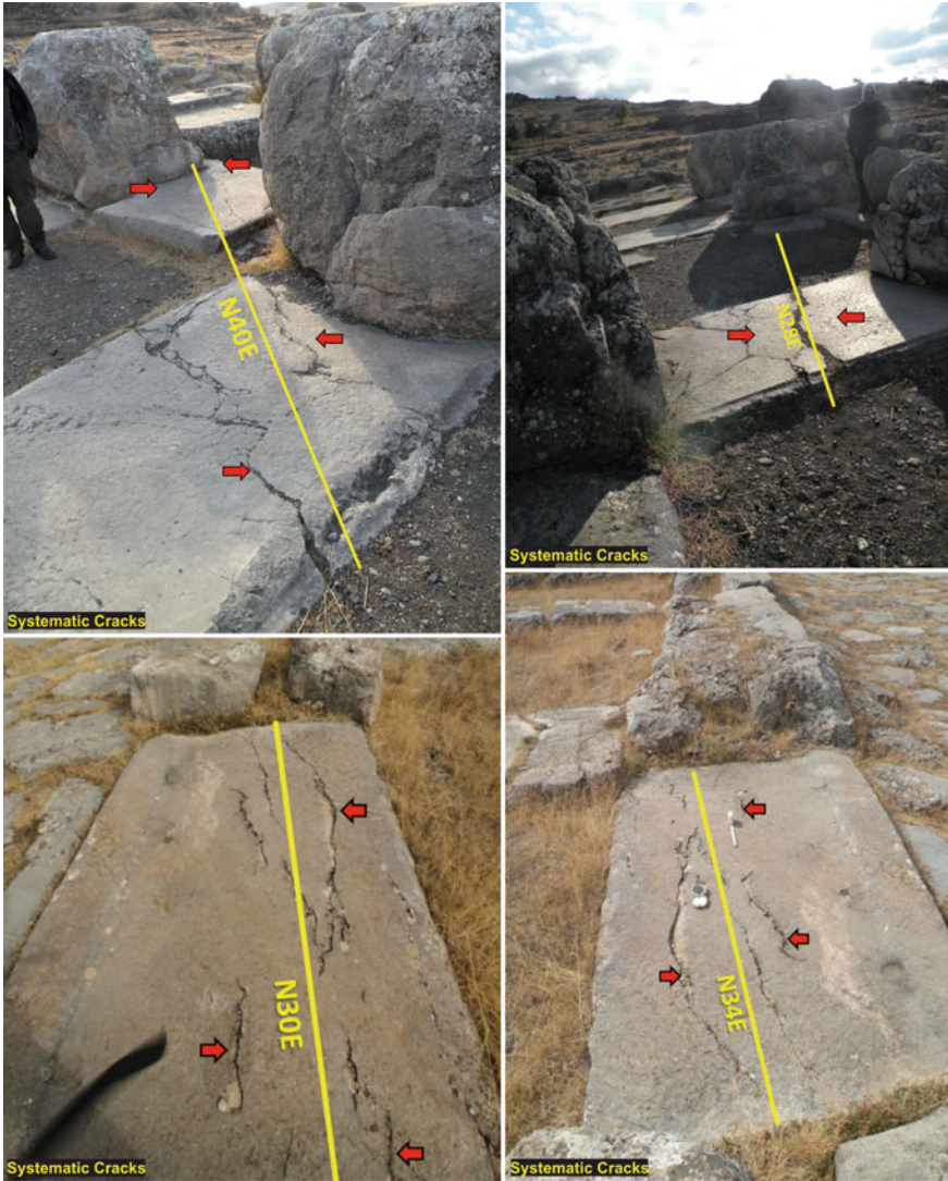
Fig. 23 NE-trending systematic cracks observed on the Great Temple and the magazine section of the Lower City
