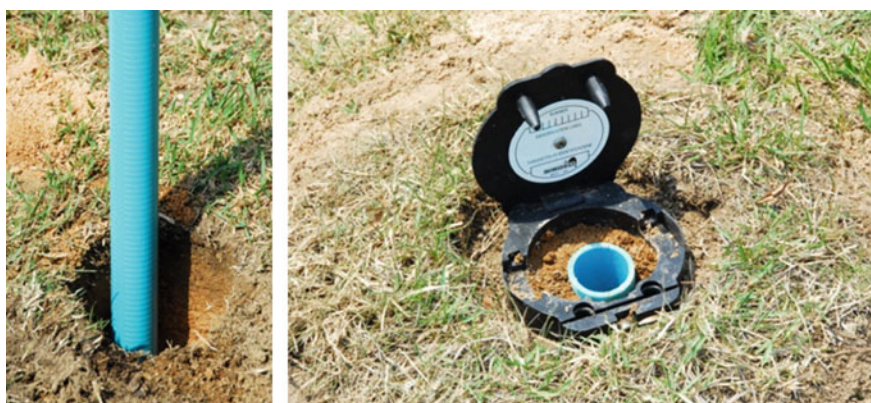
Fig. 6 The open standpipe piezometer during placing in the borehole and final installation
