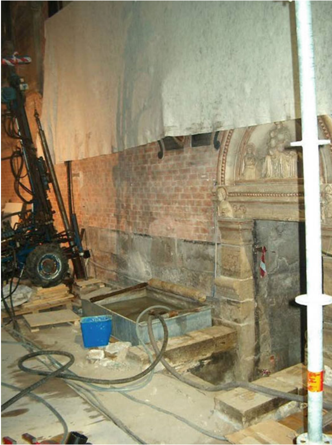
Fig. 10 Inclined borehole carried out from inside the Basilica to investigate the foundation block of the Frari bell tower as well as the subsoil below it
