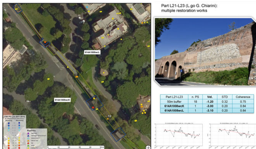
Fig. 9 Displacement due to the presence of unstable multiple restoration works
