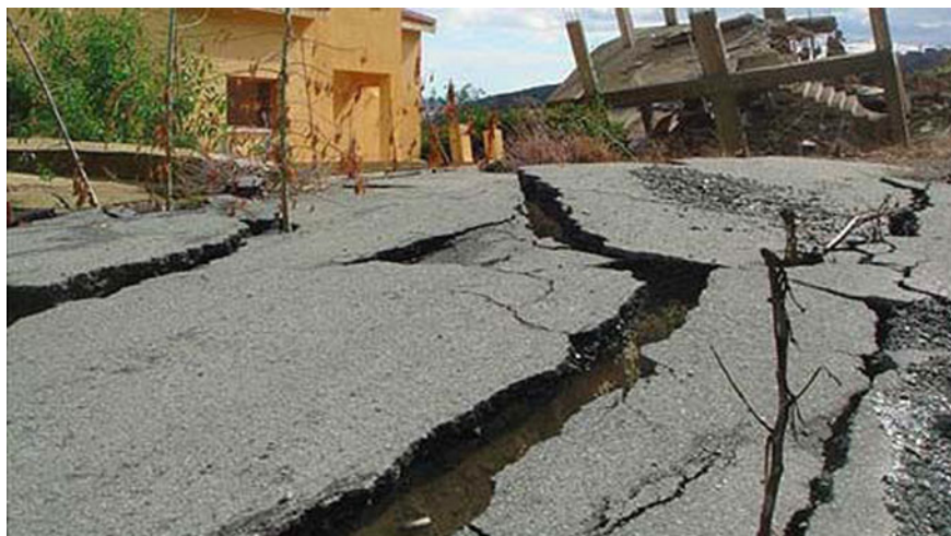
Fig. 3 Landslide in Pissouri area in Cyprus
