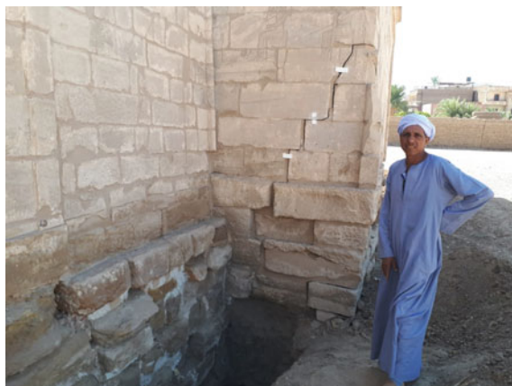
Fig. 3 One of the crack systems initiated on walls of chapels
