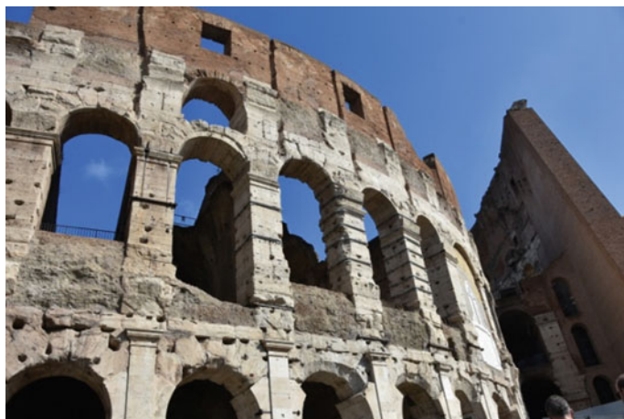
Fig. 17 Detail of pillar wrapping in the monitored area in 2020 (Parco archeologico del Colosseo, photo of D. Spizzichino)
