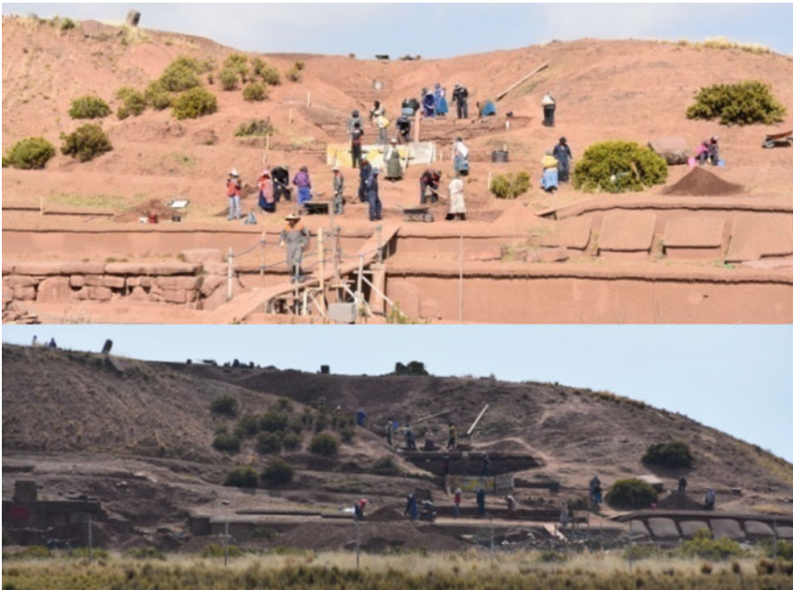
Fig. 20 The final position of gabions level and earth platform were decided jointly with local authority
