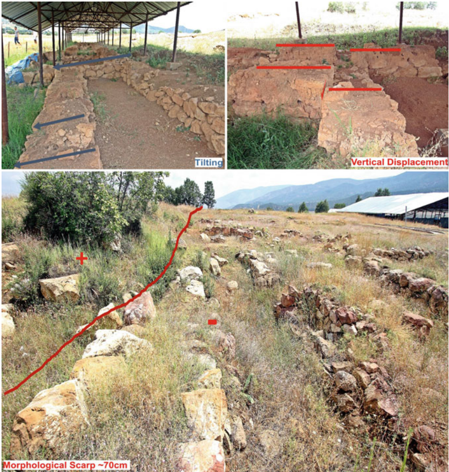
Fig. 9 Deformational structures on the building “C” and its surrounding, tilting, vertical displacement on the building wall and morphological scarp
