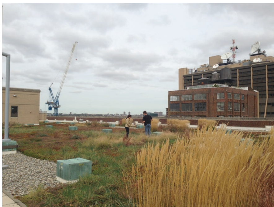
Fig. 10.3 United States Postal Service Morgan Center Processing Plant Sedum sp. green roof showing considerable contamination of non- Sedum grasses
