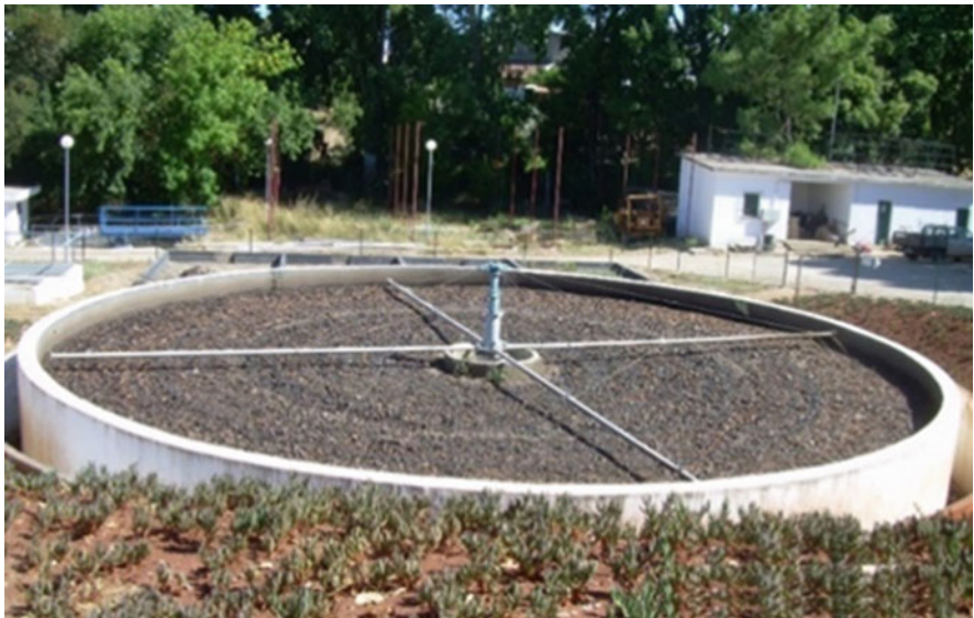
Fig. 18 Photograph of tickling filter view
