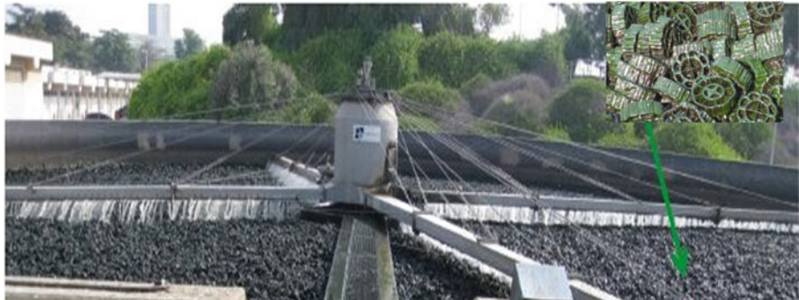
Fig. 5 Existing filter media filling in trickling filter before re-habitation WWTP-Alaweer
