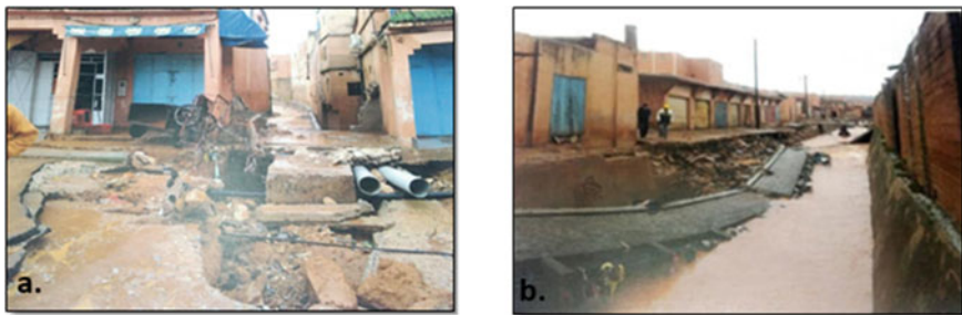
Fig. 18.1 Damage to the infrastructure of the village of Lakhssas during the floods of November 2014. a degradation of the National Road No.1; b deterioration in the inter-provincial roads connecting Lakhssas village and Ifni city
