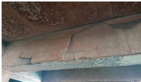
Fig. 2 Flexural cracks in beams
