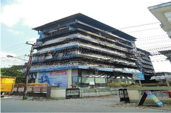
Fig. 1 Fire damaged building
