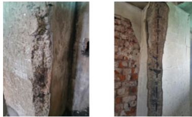
Fig. 6 Spalling of concrete on columns
