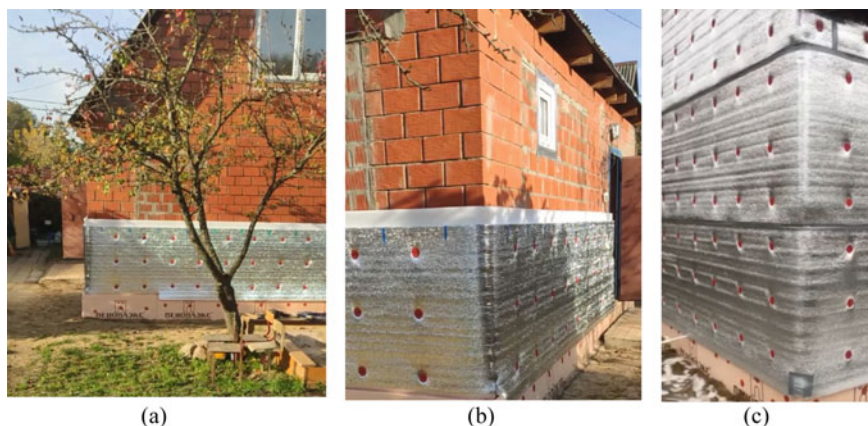
Fig. 6 Insulation with rolled polyethylene: a - the facade of the building, b - the corner of the building; c - finished insulating shell
