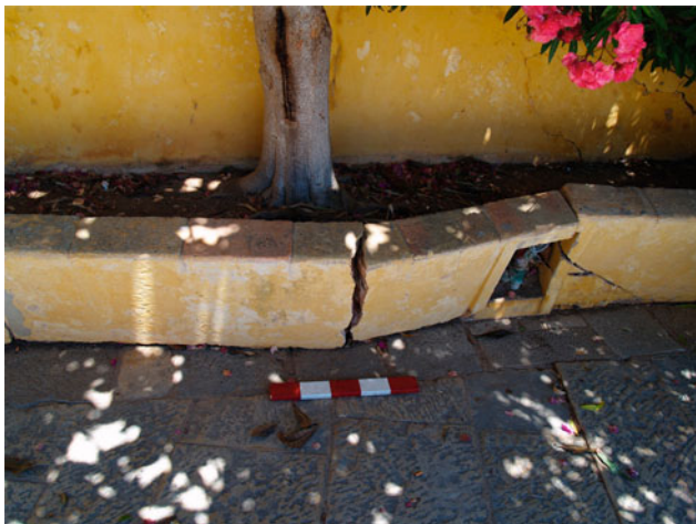
Fig. 7 One of the flowerbeds is destroyed and in risk of falling. Photograph taken by the author in August 2021
