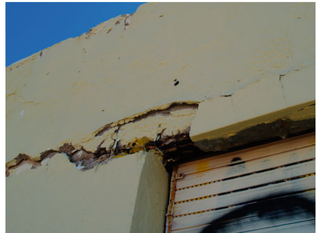
Fig. 9 Reinforced concrete applied in the 60s is already broken and eroded. Photograph taken by the author in August 2021
