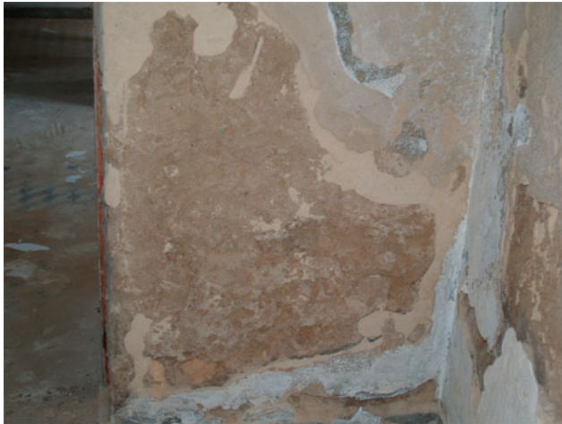
Fig. 6 In the old post of the Fiscal Guard, it is possible to see some fallen plaster. Photograph taken by the author in August 2021
