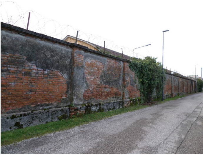
Fig. 3. Abandoned “Tommaso Salsa” barracks as urban enclave, Treviso (IT). The perimeter wall of the military site. Source: photo by F. Camerin.
