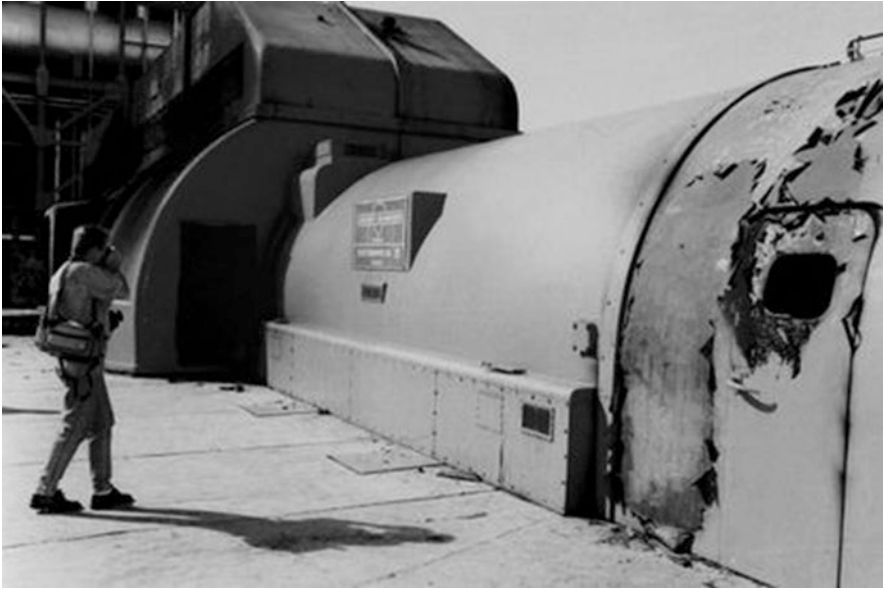
Photo 2.8 Photo taken outside (shadow of the photographer) probably showing a fan motor cowling damaged by the fire (photo J.L. Sellart)
