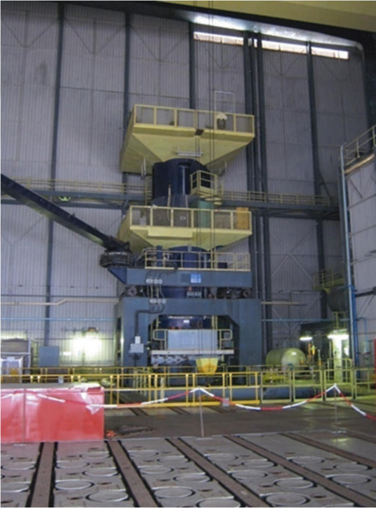
Photo 2.81 Natural uranium graphite gas reactor (first French reactor type). The Saint Laurent-A loading platform and the Main Handling Device (DPM). The rails of the fuel loading machine and the tulip-shape plugs (with circular top) closing the CO 2 channels are visible in front of the photograph (photo: Bouchacourt-Foissote-Valdenaire-ENSIB)
