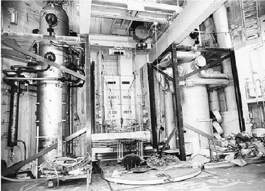
Photo 2.66 The floor at SGs level after the accident
