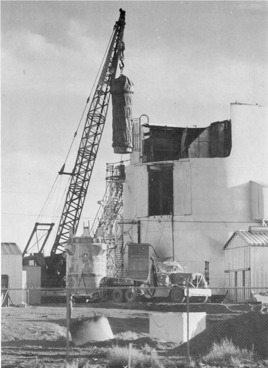
Photo 2.35 Extraction of the vessel through the reactor dome with a mobile crane. A trailer truck carries a transport cask for the vessel
