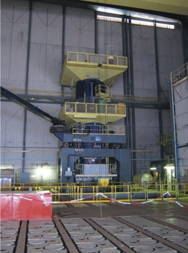
Photo 1.3 Natural uranium graphite gas reactor (first French reactor type). The Saint Laurent-A loading platform and the Main Fuel Handling Device. The rails of the fuel loading machine and the tulip-shaped plug closed next to a CO 2 channel can be seen (photo: Bouchacourt-Foissote-Valdenaire)
