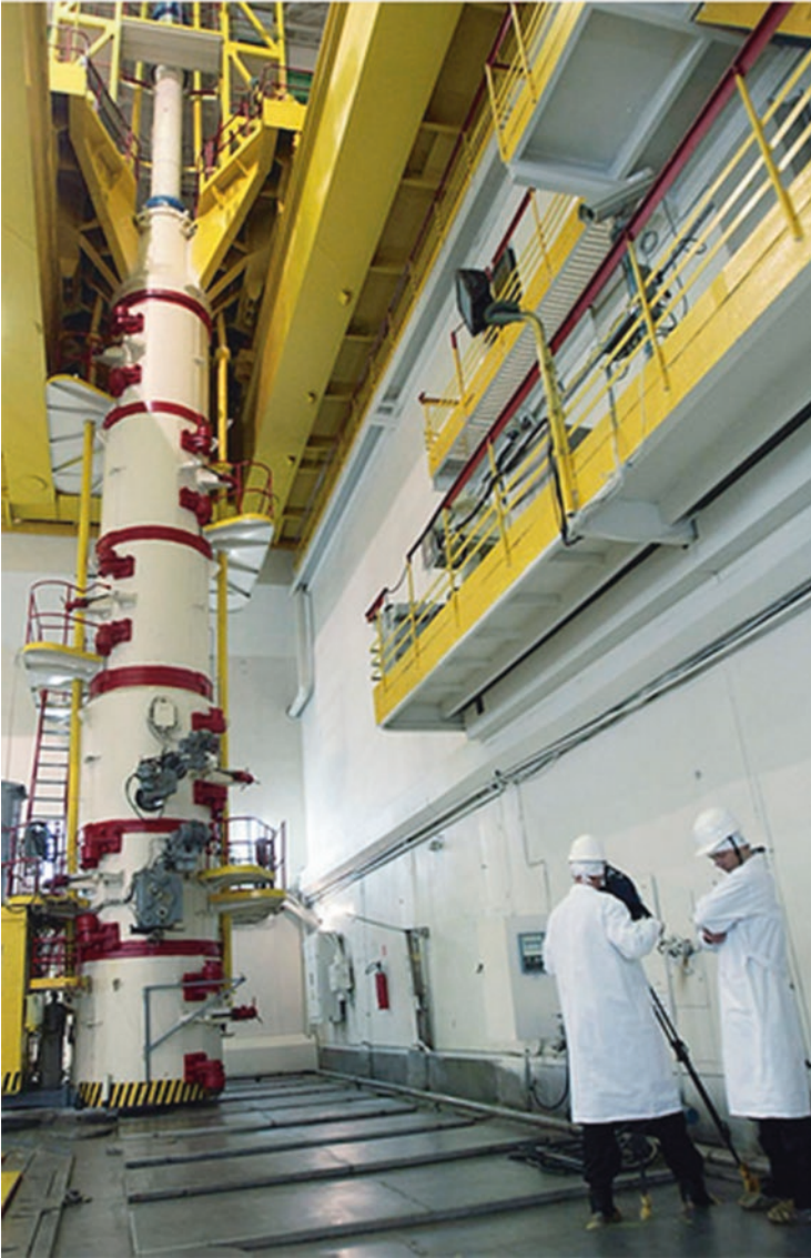
Photo 4.22 Assembly handling system. The very large size of the system is due to the height of the assemblies (almost 7 m!)
