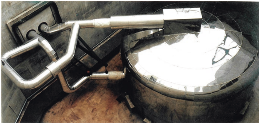
Photo 1 Principle and photo of a U5 filter of a P4 unit (photo EDF). The aerosols arrive at the top of the filter and the non-retained volatile gases are evacuated through the lower pipe toward the TEG stack. The filter can be bypassed in case of severe blockage
