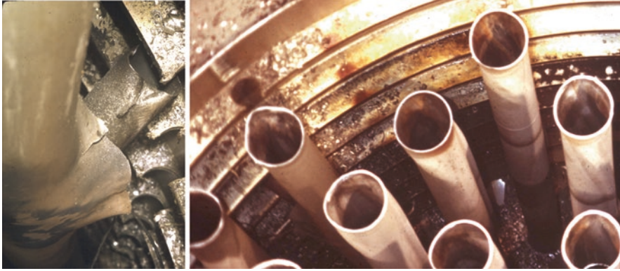
Photo 2.71 Double connection of channel 59 (left) and channel deformation (right)
