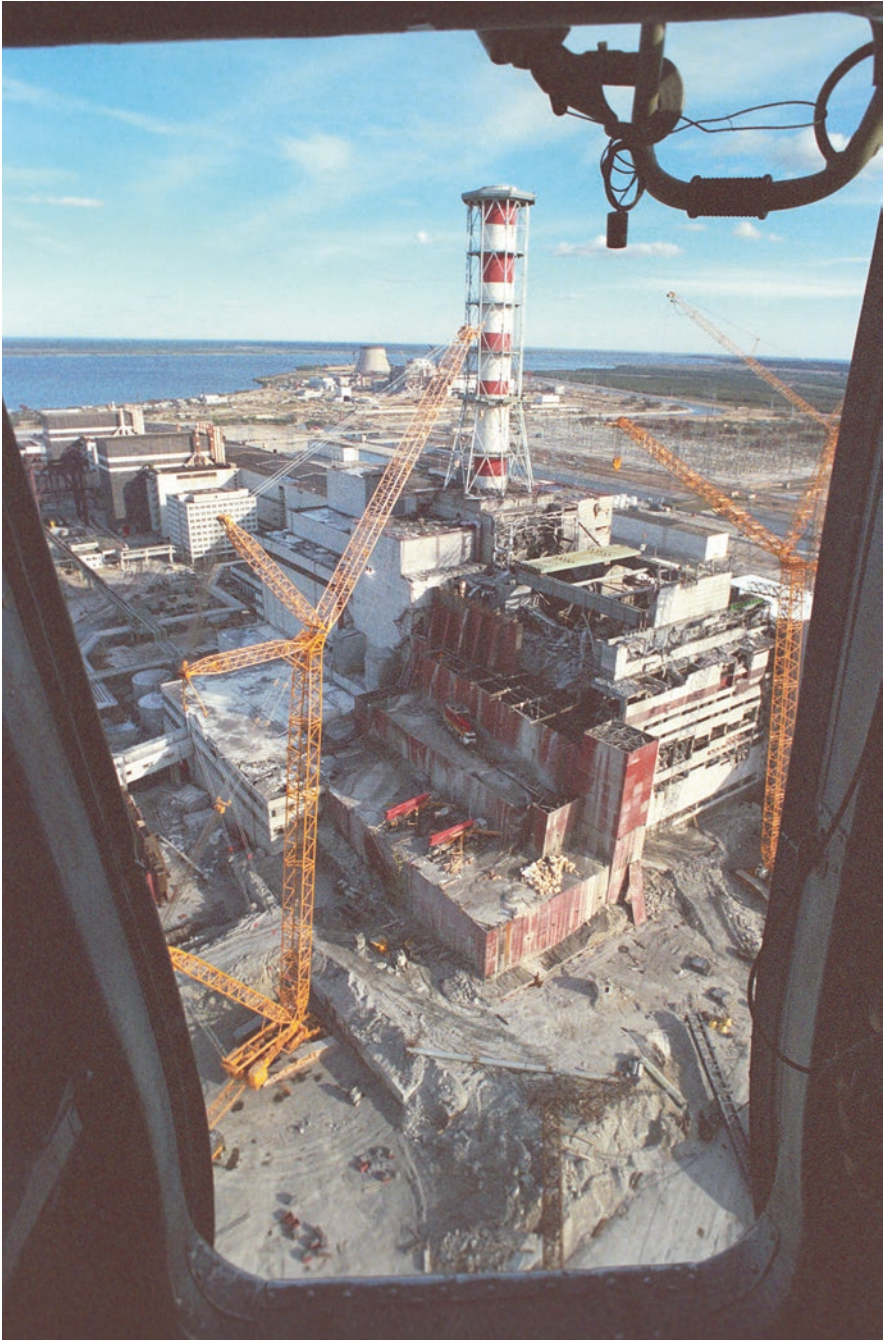
Photo 4.10 An impressive photo taken through the open door of a helicopter, during the construction of the first sarcophagus (photo DR). A truck, which one wonders how it arrived there, gives the measure of the whole picture
