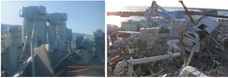
Photo 5.5 Damage on the seawater pumps: unit-3 (left) and unit-5 (right) (photos TEPCO). One can see the immediate proximity of these pumps to the sea by their function. The dam was ineffective to protect them
