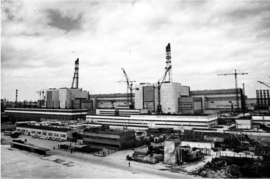
Photo 4.3 Construction of the two Ignalina reactors in Lithuania in the early 1980s
