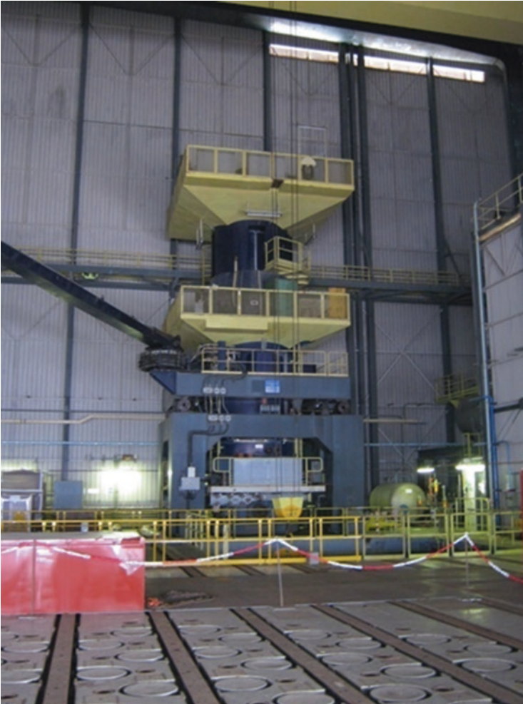
Photo 2.81 Natural uranium graphite gas reactor (first French reactor type). The Saint Laurent-A loading platform and the Main Handling Device (DPM). The rails of the fuel loading machine and the tulip-shape plugs (with circular top) closing the CO 2 channels are visible in front of the photograph (photo: Bouchacourt-Foissote-Valdenaire-ENSIB)
