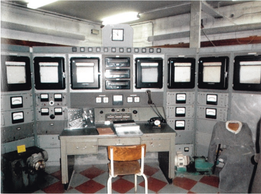
Photo 2.19 The same control room of Zoé (France) renovated at the end of the 60s. Many “head-up” recorders were installed. We can see the “Human Factors” progress brought to the control console. ZOE’s core shutdown on April 6, 1976 at 11:51 a.m. after 28 years of good and loyal service, and above all without accident! (CEA photo)
