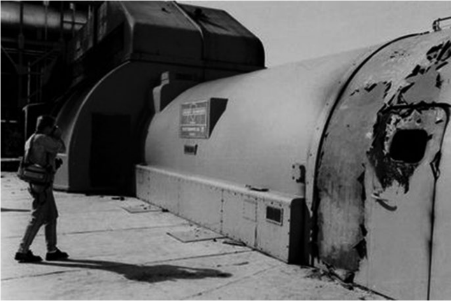
Photo 2.8 Photo taken outside (shadow of the photographer) probably showing a fan motor cowling damaged by the fire (photo J.L. Sellart)
