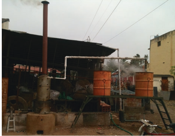
Fig. 5 View of efficient combustion system
