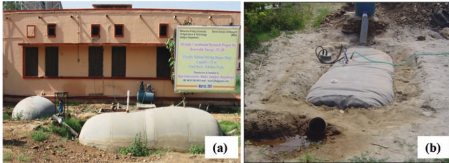
Fig. 2 View of the (a) installed prefab balloon digester; (b) installed digester
