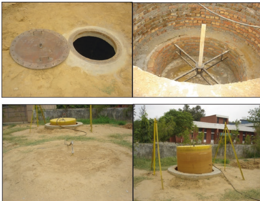
Fig. 1 Different phases of a paddy straw-based biogas plant
