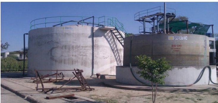
Fig. 7 Odorless bio-methanation system at Mother Dairy, FVU, New Delhi
