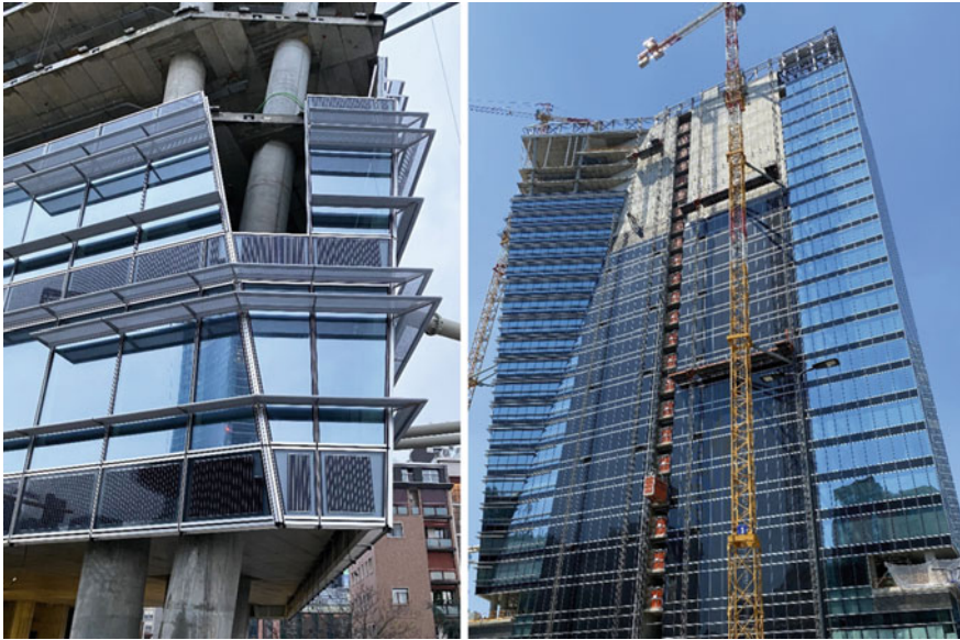
Fig. 8.3 Construction phases of GIOIA 22 tower (North/West and North/East elevation)—Crystalline Silicon glass BIPV—Gioia 22 Tower, Milan, Italy
