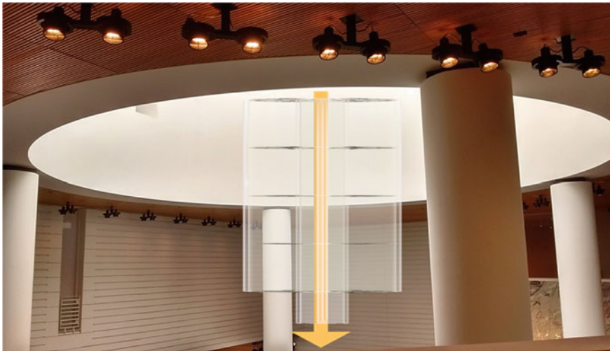
Fig. 1.7 Installation of a building solar radiator based on the concept of EFPHS
