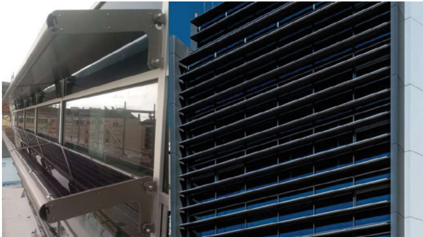
Fig. 8.14 Monocrystalline horizontal Louvers, Avenida Diagonal 525, Barcelona, Spain (courtesy of Onyx Solar)
