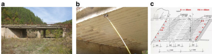
Fig. 3 a Bridge B36. b Impact testing. c XX de-bonded areas
