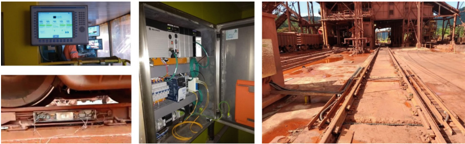
Fig. 6. DRS system environment and equipment.
