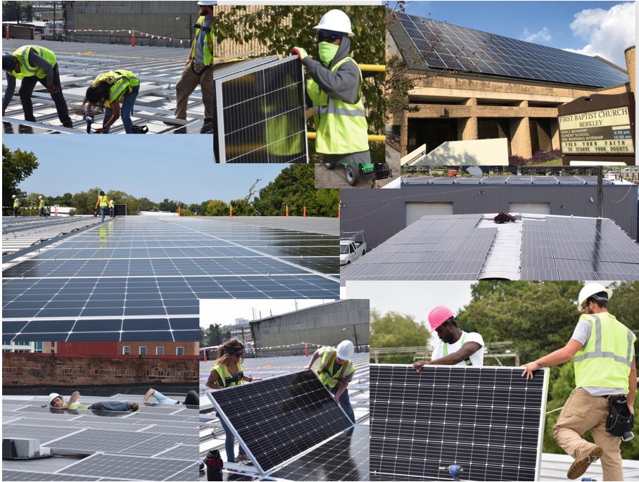
Fig. 1. Solar installations by Norfolk Solar QOZ Business.
