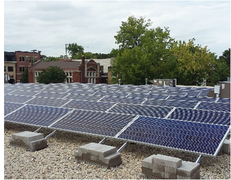
Fig. 3. The Heliene solar panels on roof
