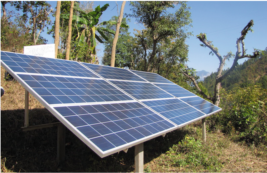
Fig. 9. SWP array rated at 1.26 kW p used for irrigation by the Taule village farmers.
