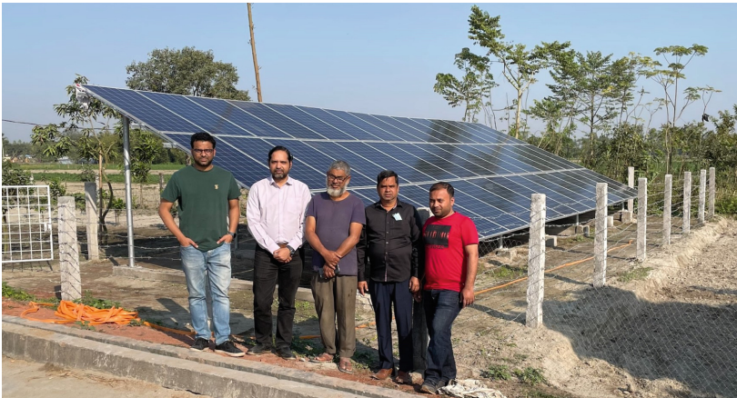
Fig. 10. Bangladesh BREB SPPAI 7.5 kW SWP installed in Dinajpur in December, 2021.
