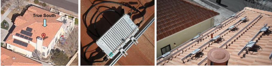
Fig. 1. 3 kW photovoltaic installation in Albuquerque, NM, using Enphase's first-generation microinverters.
